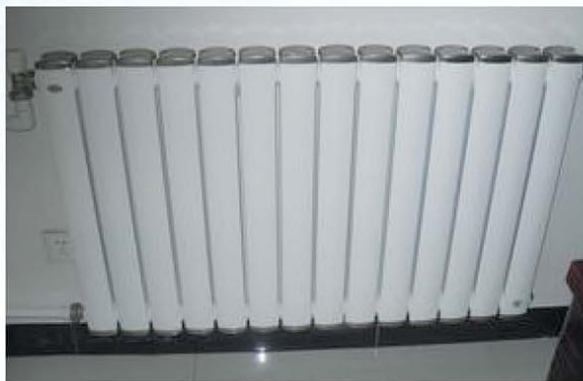
▲ water heat radiator
